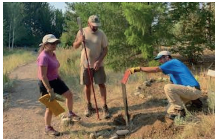
Installing signs. From left: Linda Ries, Paul Ries, and Jim Rineholt checking the straightness of the post.
